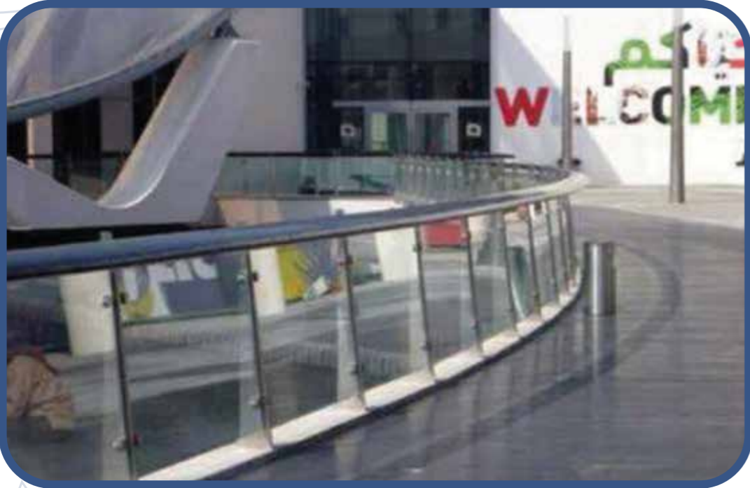
Project: Fabrication and Installation of Stainless Steel Handrails with Timber Rail Client: Citiscape (Ferrari Theme Park)/Six Construct
